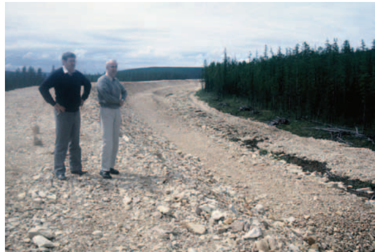
BAM railway extension under construction with embankments three to four metres high
