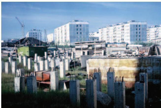
Piles for a high rise building being left for a winter to freeze into the permafrost soil.
