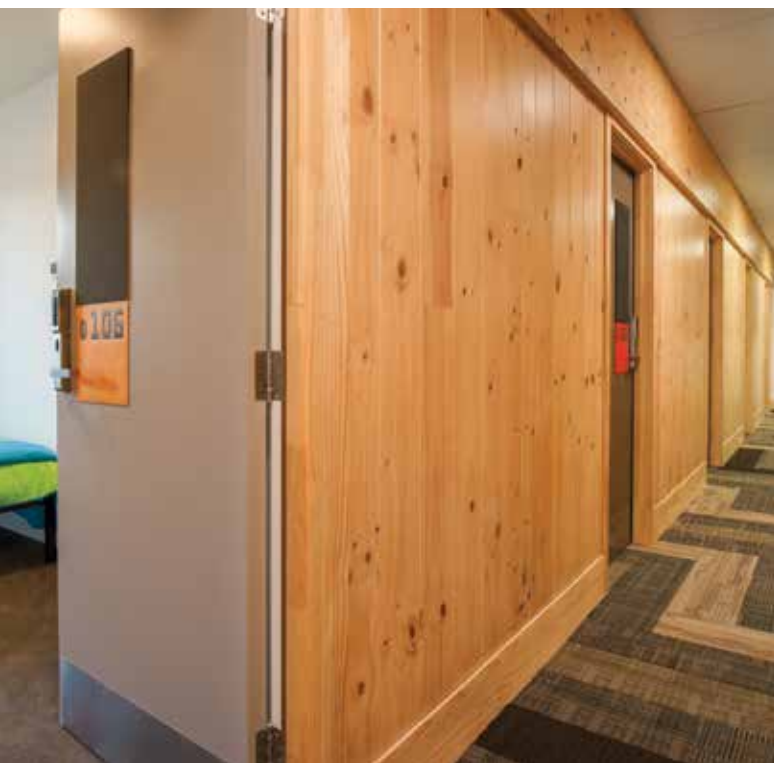
Finished project showing exposed wood features and entrance into one of the many student accommodation rooms. Photo courtesy of Logic Group
