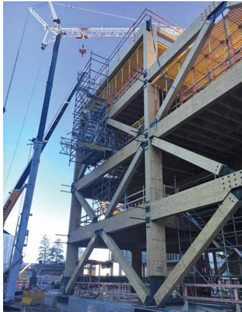
The Beatrice Tinsley Building at the University of Canterbury under construction. An academic support building in the new Rutherford Regional Science and Innovation Centre, it uses LVL and is a Jasmax large-scale timber project. Photo courtesy of Jasmax
