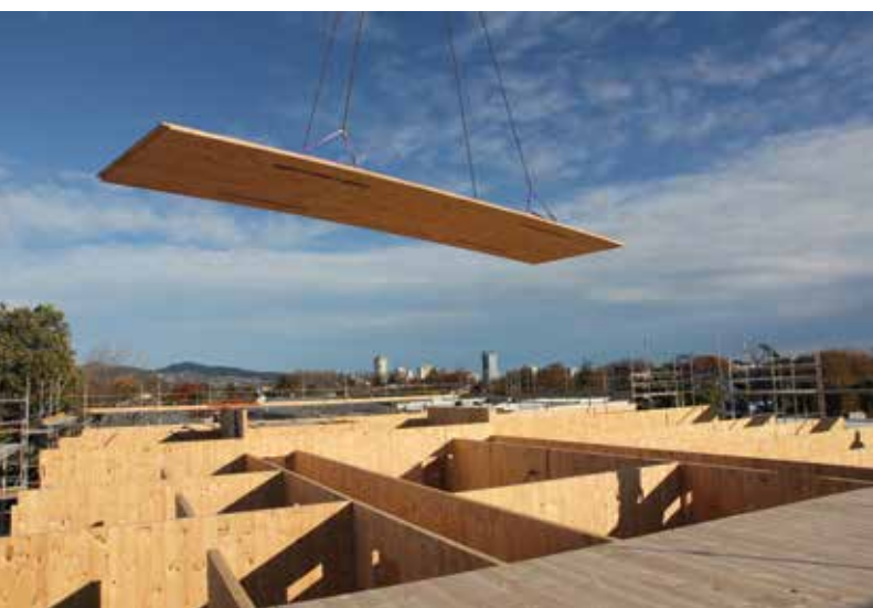
Bealey Lodge, Christchurch, under construction. The speed and accuracy of CLT buildings becomes very visually apparent when the buildings go up much faster than traditional materials in commercial buildings. Photo courtesy of Engco
